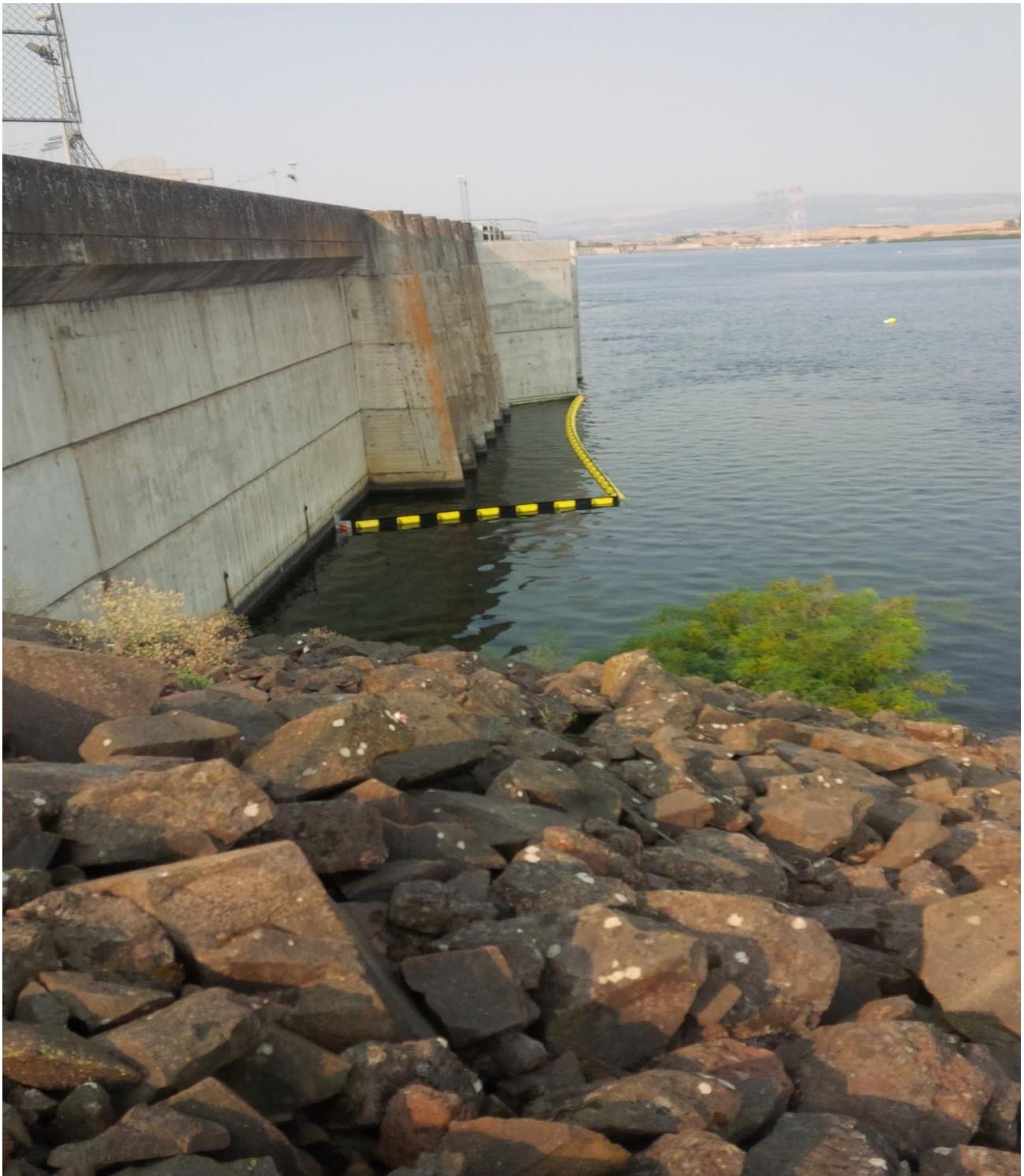
Newly installed permanent boom forebay of east fishladder to protect from upstream oil spills.
